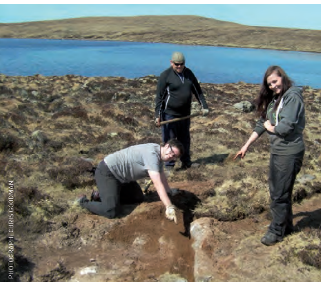
Students from Fife's Elmwood College work on repairing a section of the Sandwood path
